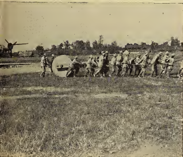
A Chinese labor army employs primitive methods to construct an airfield at an advanced base.
